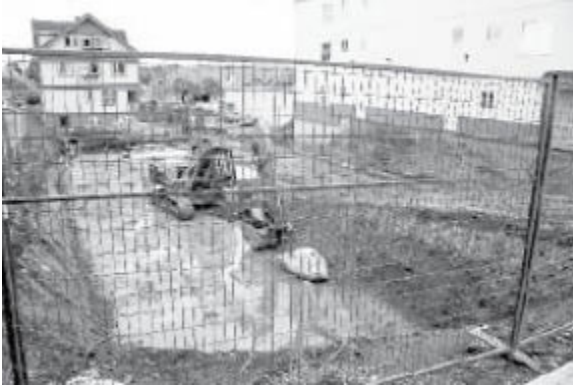
Gurcharen Budwal bucks the Victoria trend and sets to work on a new apartment building on Pembroke Street
